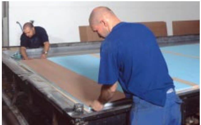
Fig. 8 Once the adhesive has been applied, a laminated wooden layer is installed
